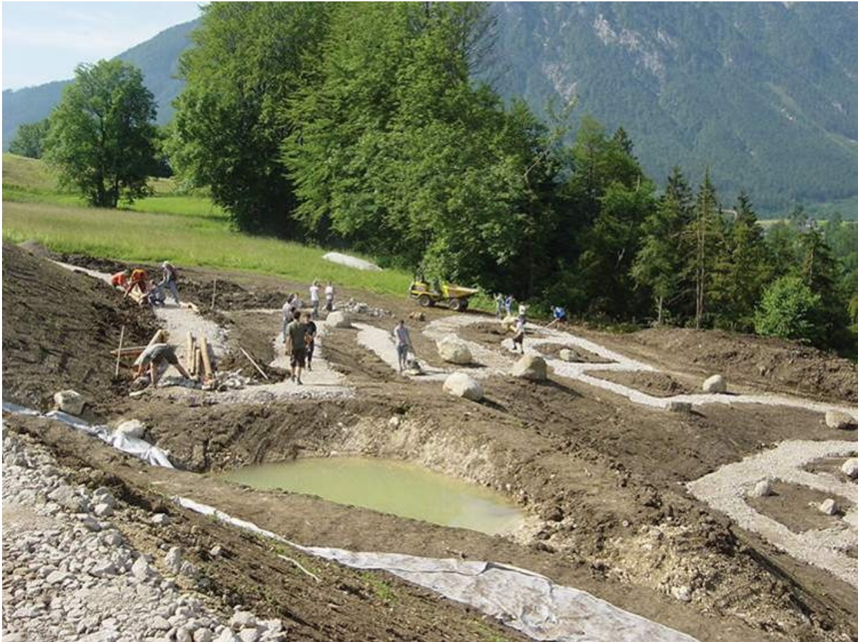
The structure of the sensory garden: the remaining work mostly needs to be carried out by hand.
