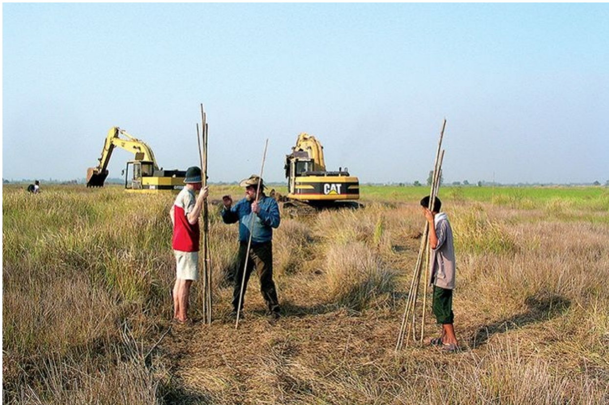
The edges of the letters are marked with poles, so that work with the excavator can begin.
