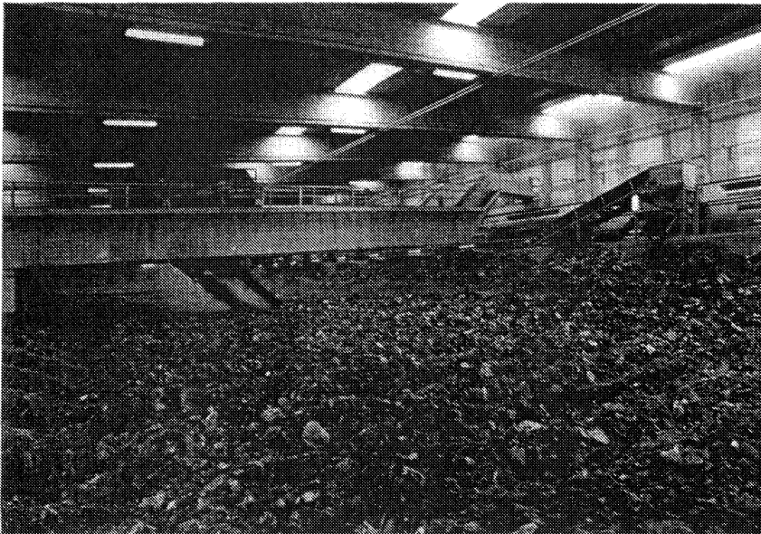
Figure 2.31. Sorain Cecchini agitated bin system composting pre-processed MSW at Perugia, Italy. Material is loaded along one side of the bin length (right side in photo), moves across the bin width by action of the agitation screws, and is discharged at the opposite side. Four agitation screws are mounted on a 30 m traveling bridge. The screws move along the traveling bridge while it is stationary (from left to right in photo). Each cycle is about 15 min long. At the end of each cycle the screws retract and the bridge moves a few meters in the direction of the basin length. The bridge takes about two working shifts to run the entire 120 m basin. Photo courtesy of John Nutter, Sorain Cecchini Recovery.
