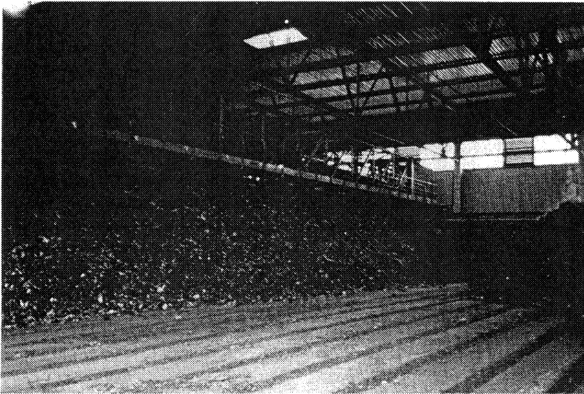
Figure 15.8. Permanent, parallel manifold channels in the floor of a refuse composting hall. Each aeration channel is rectangular in shape and is covered by wooden blocks. Gaps between the blocks serve as orifices to collect the gases that flow by downward, induced draft. Site is the Siggerwiesen co-composting plant serving the City of Salzburg, Austria.
