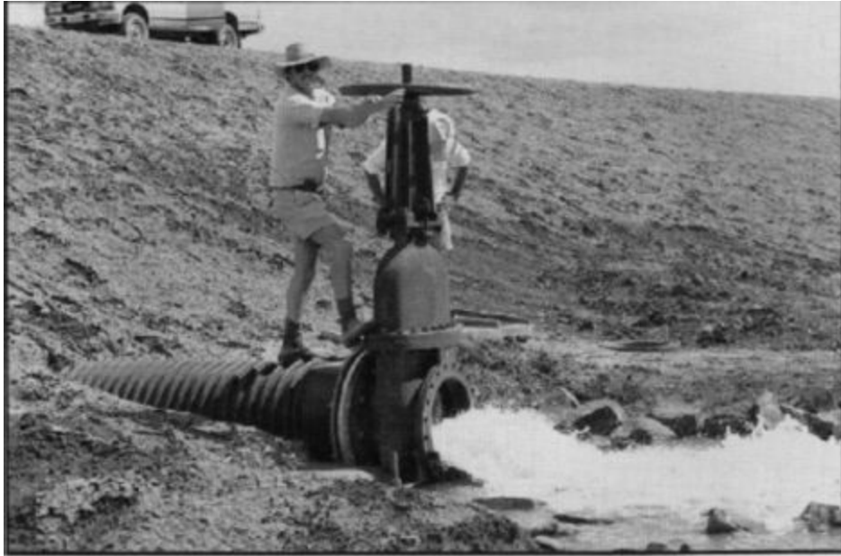
Plate 9 First flow from an irrigation dam. 600 mm (2 feet) diameter pipe with a slightly undersize valve. Maximum flow is about 3.5 m 3 /sec., which is 12.6 ML/hour and 10 acre feet per hour. Irrigation application rate is up to 20 ha (50 acres) per hour.
