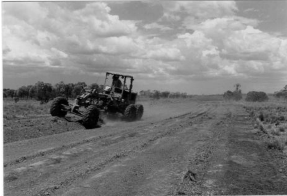
Plate 43 A Main Flood-flow irrigation channel under construction. The dam can be glimpsed in the background.
