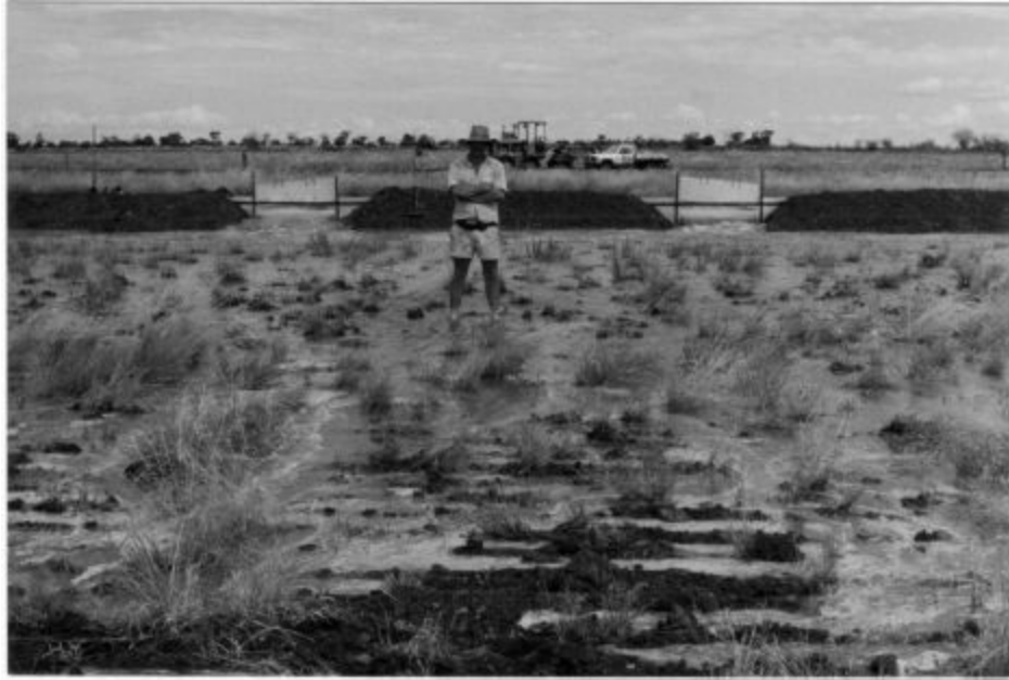
Plate 49 First flow into an irrigation bay. Without ripping most of the water would run off but here the water quickly pours into the loosened soil.
