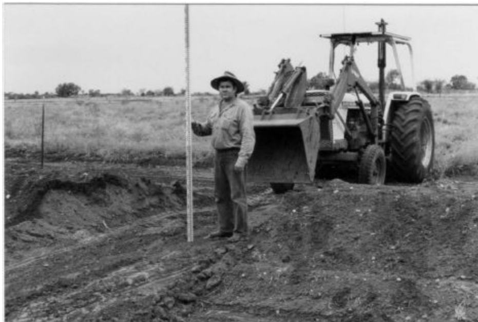
Plate 46 Checking the level of the cut through the bank prior to installing the watergate.
