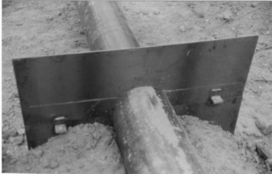
Plate 27 Earth filled to half way up the pipe ready for final pass of hand ramming.
