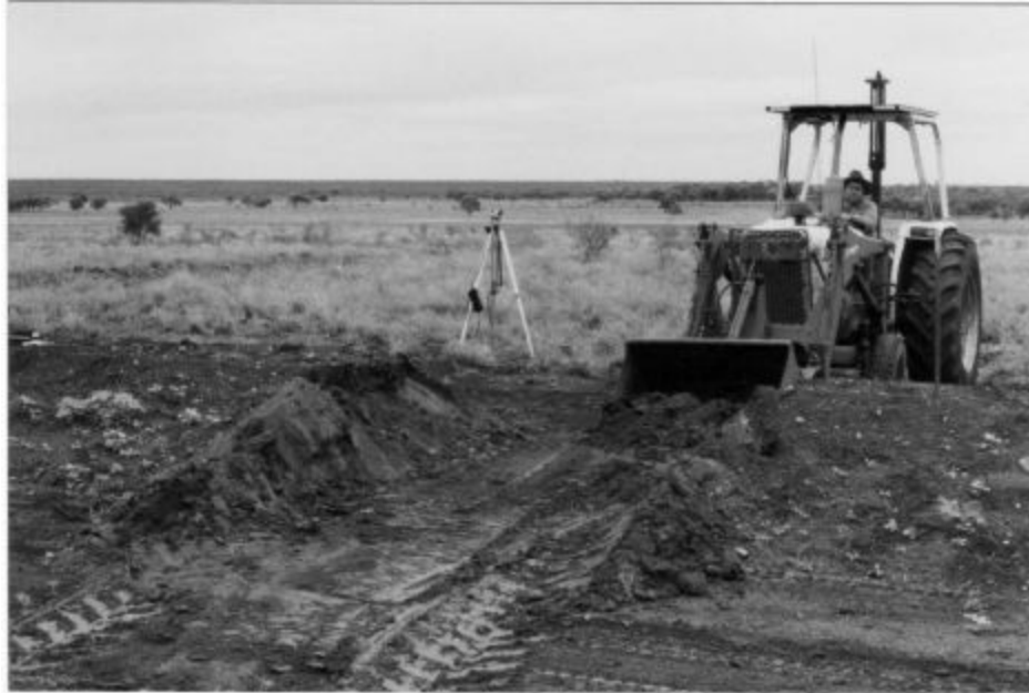
Plate 45 A front end loader is used to remove a section of a Flood-flow irrigation channel's bank for the installation of a water gate.
