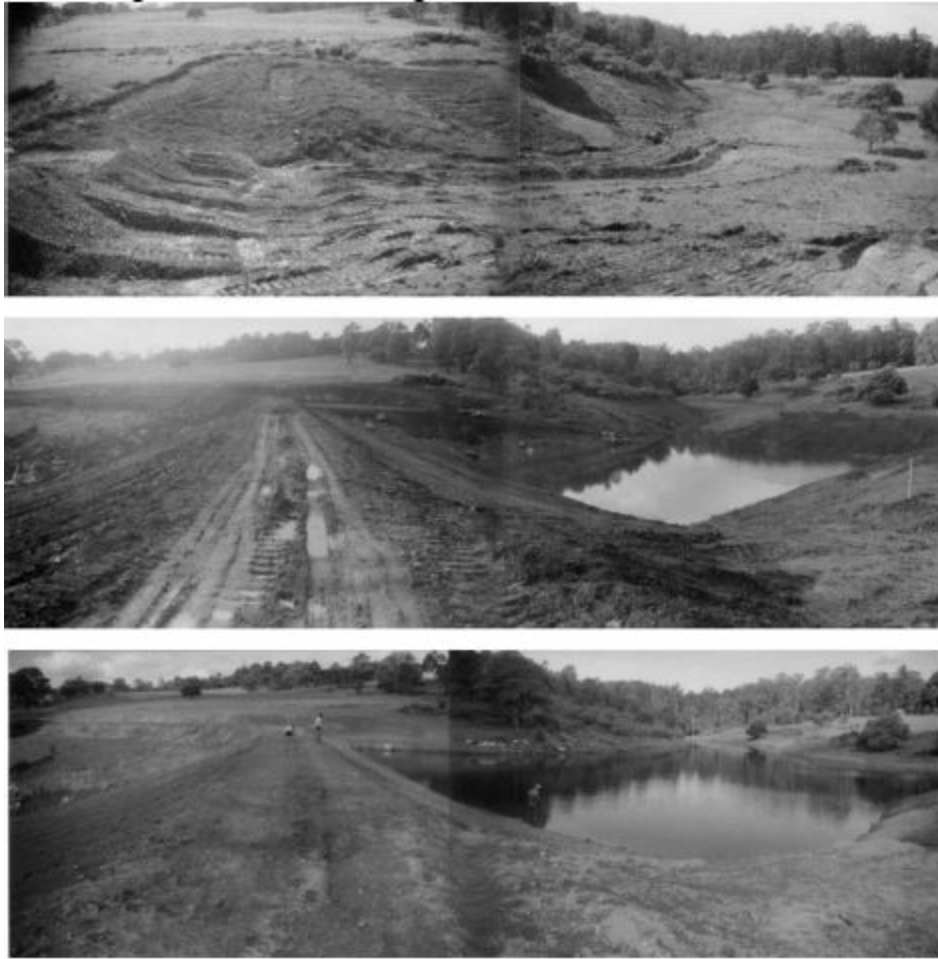
Plate 5 Construction sequence of an on farm irrigation dam near Armidale NSW. The Lockpipe enables direct gravity irrigation and feeds a pump to an upper irrigation dam in the trees at top left.
