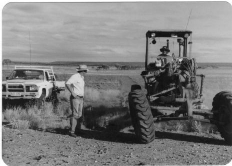
Plate 51 The first of two passes with a grader in the construction of a steering bank.
