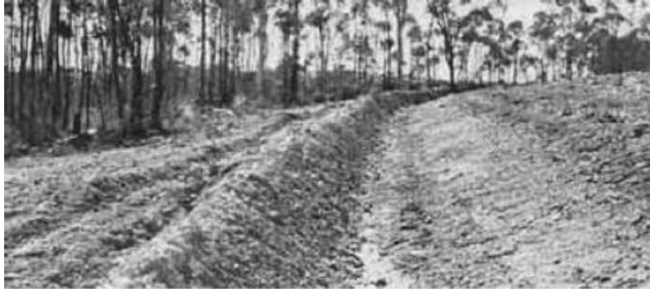
Plate 39 Early (1958) feeder channel constructed by bull dozer. Note parallel belt of timber left below the channel.
