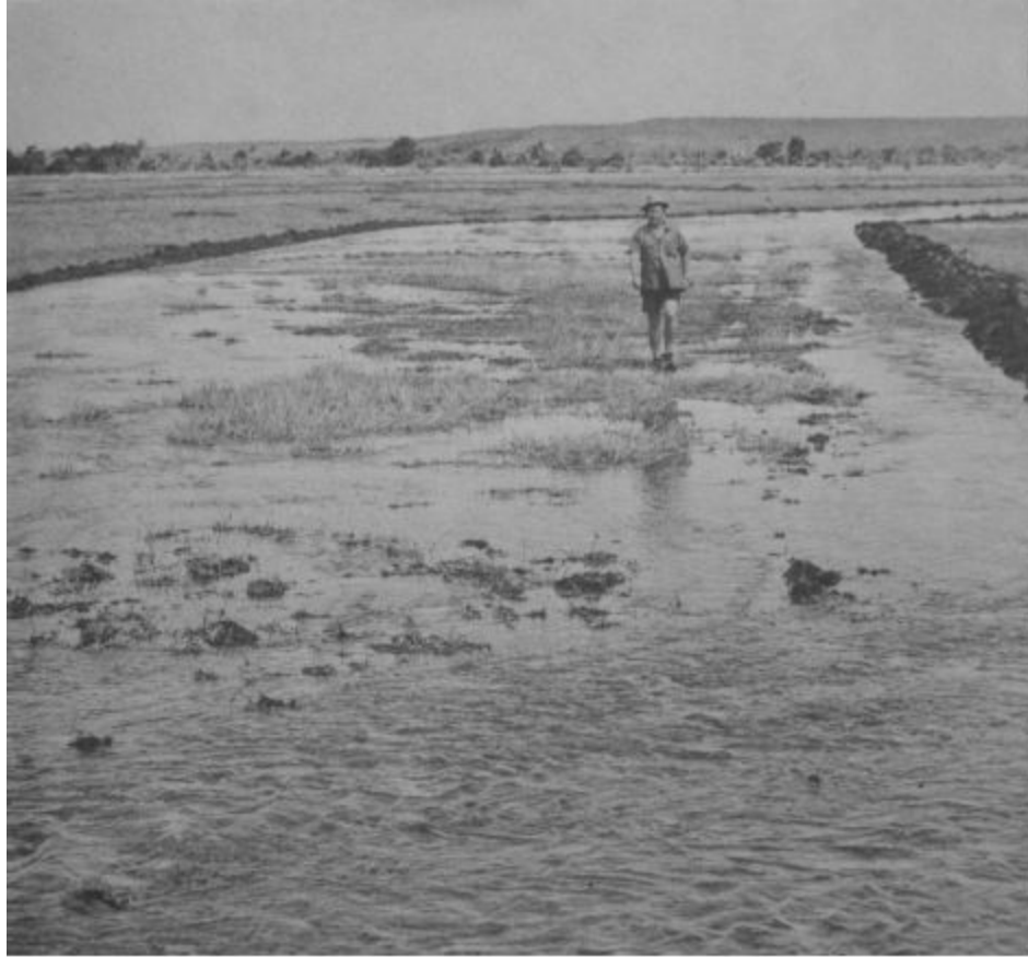
Plate 42 Looking along the contour of a dual bank Flood-flow irrigation channel. The first test flow of 1.8 ML/hr in a channel designed to carry 9 ML per hour (2,000,000 imp gal/hour).
