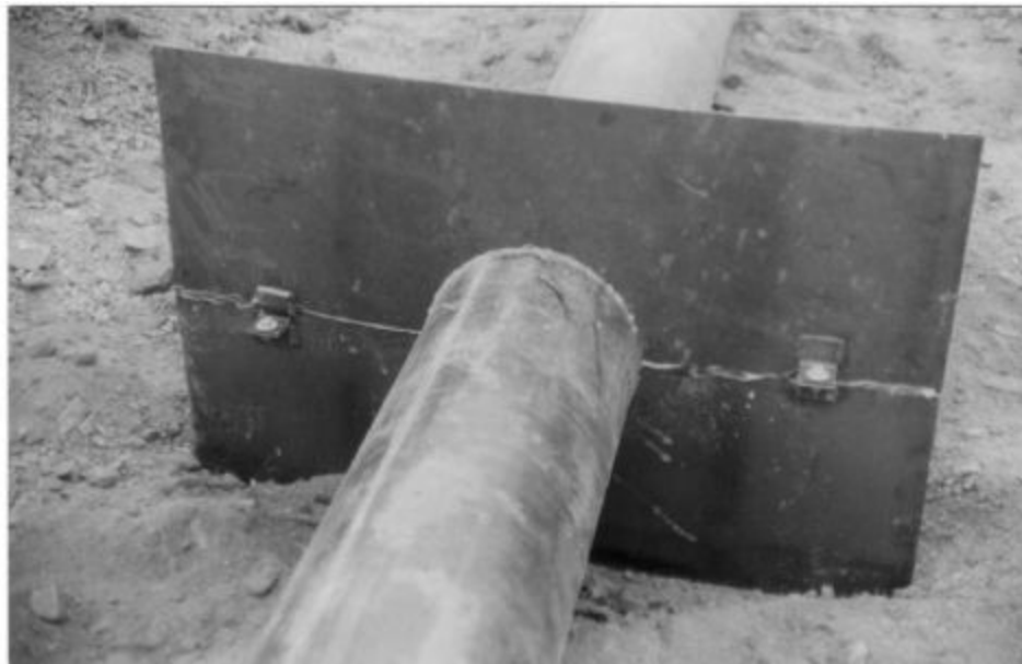
Plate 25 Baffle plates prevent water from flowing along the outside of the pipeline under the dam wall. They are bolted in place. The use of a sealing compound around the pipe and between the baffle plate halves prevents seepage.
