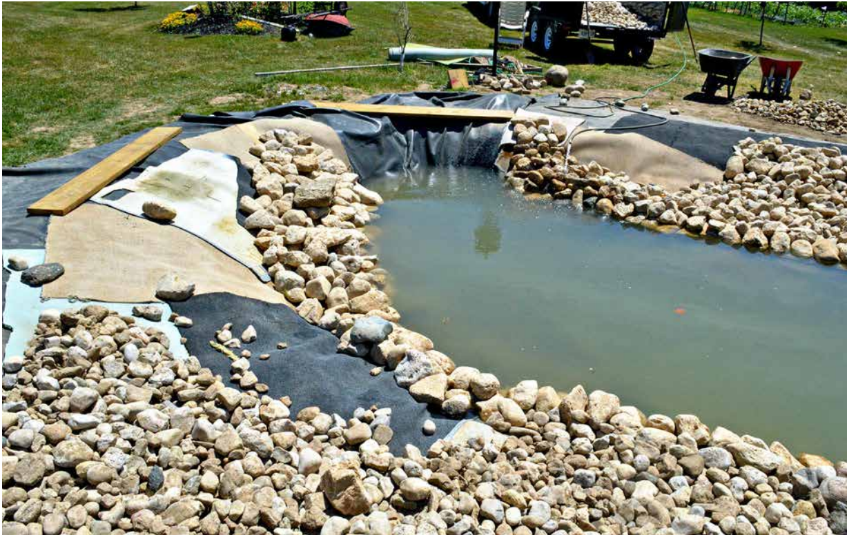
FIGURE 23 Carpet has been used as the overlayment to prevent punctures from above the liner.
